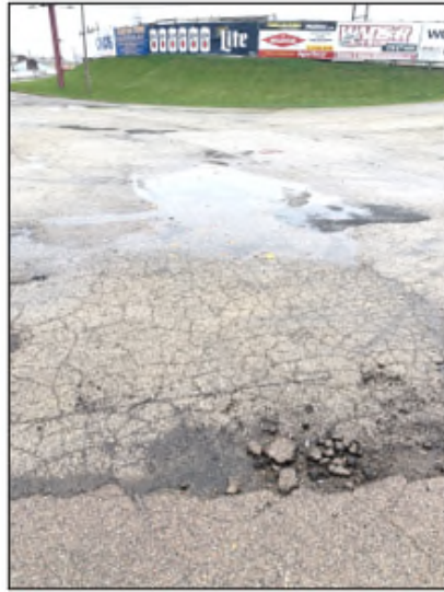
Deteriorated pavement on the Speedway property
