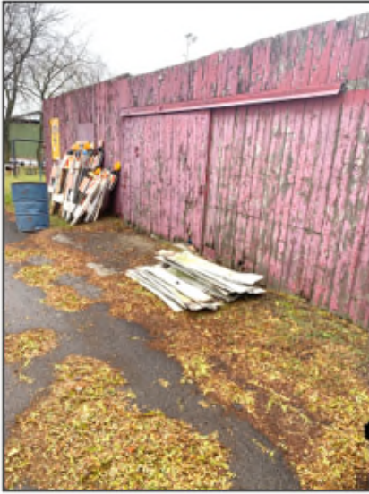
Deteriorated storage structure on the Speedway property
