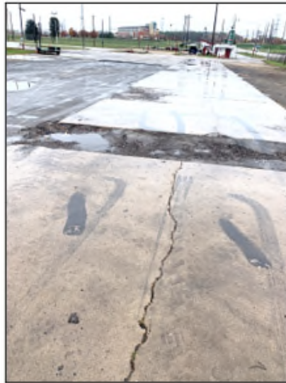
Deteriorated pavement on the Speedway property
