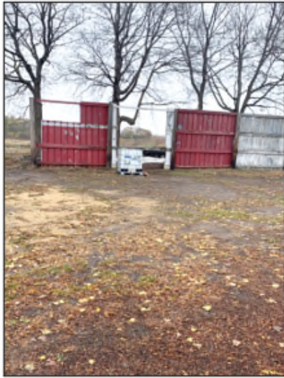
Deteriorated fencing on the Speedway property
