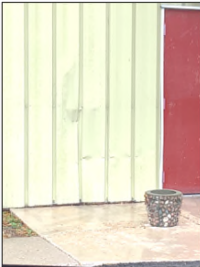
Deteriorated siding on structure on the Speedway property
