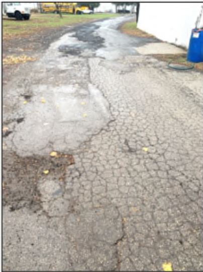
Deteriorated internal drive on the Speedway property
