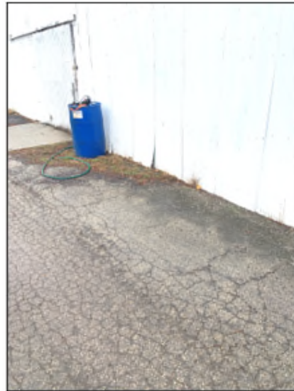
Deteriorated storage structure on the Speedway property
