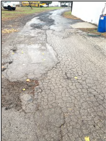
Deteriorated internal drive on the Speedway property
