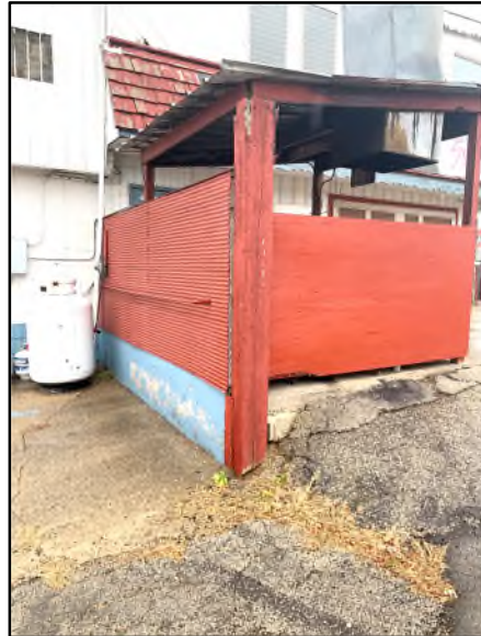
Deteriorated awning and structure on the Speedway property
