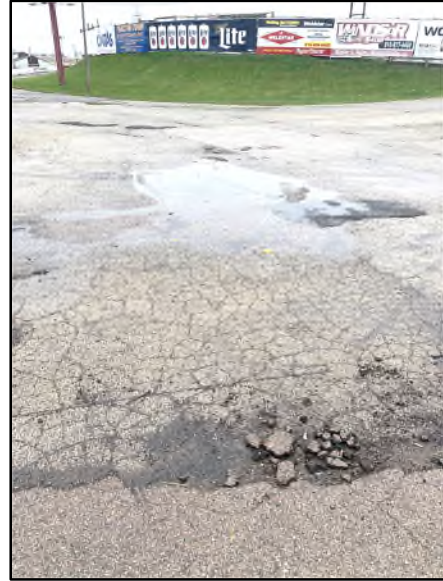
Deteriorated pavement on the Speedway property
