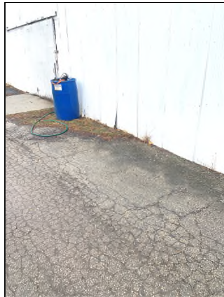
Deteriorated storage structure on the Speedway property
