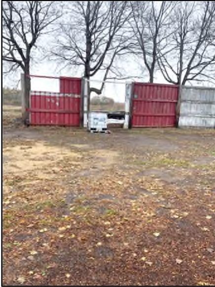
Deteriorated fencing on the Speedway property
