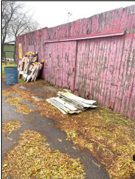
Deteriorated storage structure on the Speedway property
