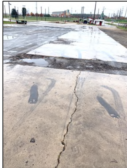
Deteriorated pavement on the Speedway property
