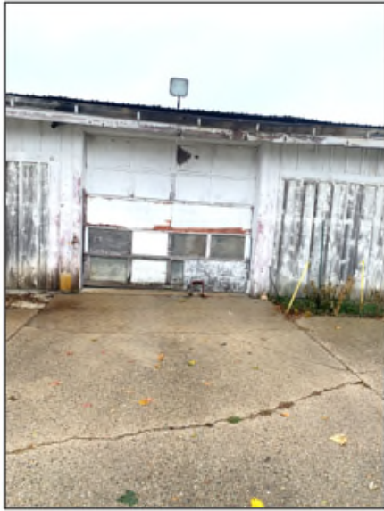
Deteriorated structure at 4191 McFarland Road
