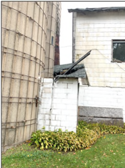
Deteriorated and dilapidated structure at 4191 McFarland Road
