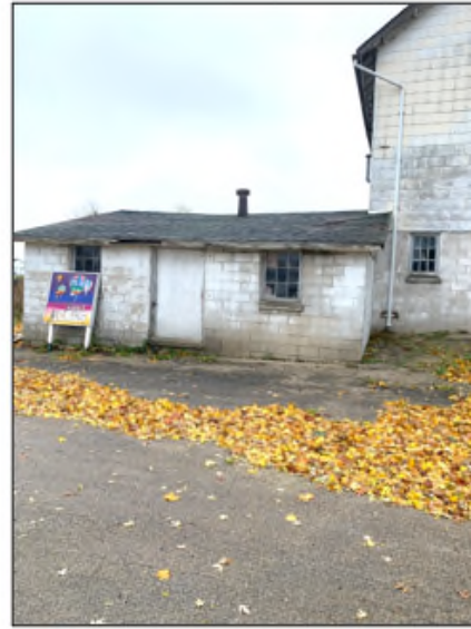
Deteriorated windows and roof on structure at 4191 McFarland Road
