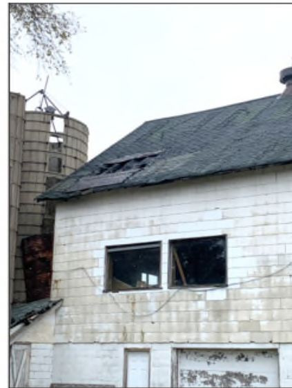
Deteriorated structure at 4191 McFarland Road
