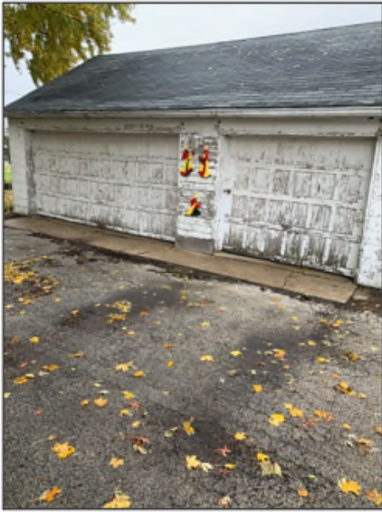
Deteriorated structure at 4191 McFarland Road
