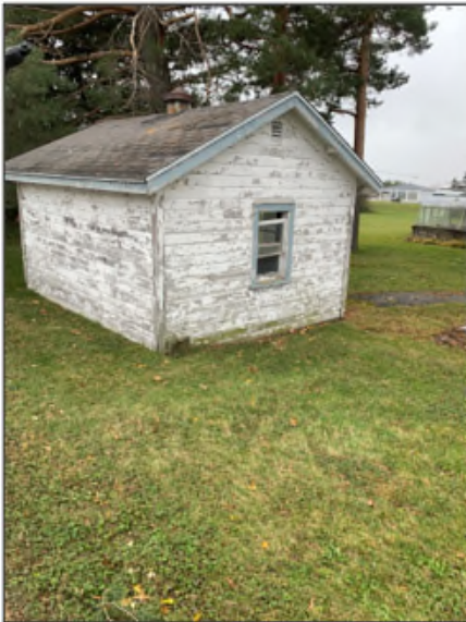
Deteriorated structure at 4191 McFarland Road
