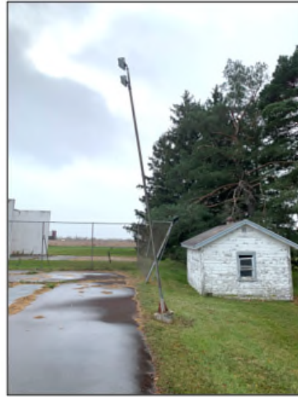
Deteriorated fencing at 4191 McFarland Road
