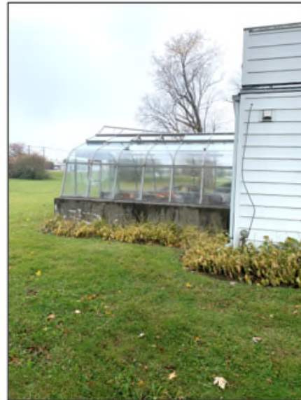
Deteriorated roof on structure at 4191 McFarland Road
